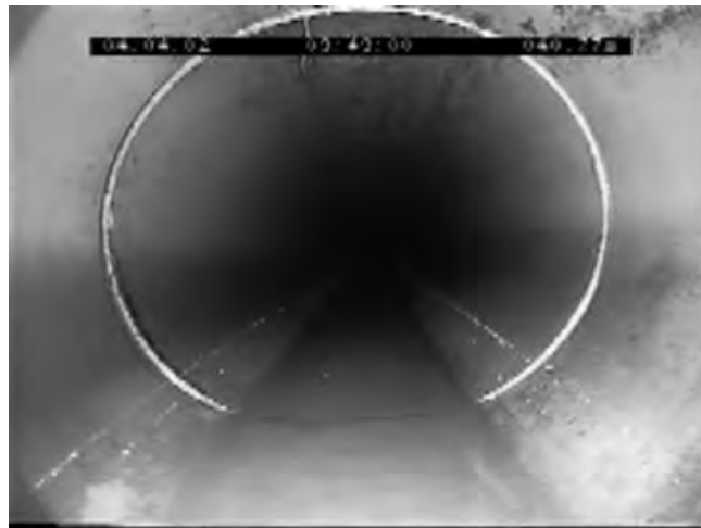
Fig.12. The deflection of the top of the pipe in the 4th class of failures
