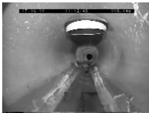
Fig. 16. The house sewer that juts out to the pipe interior
