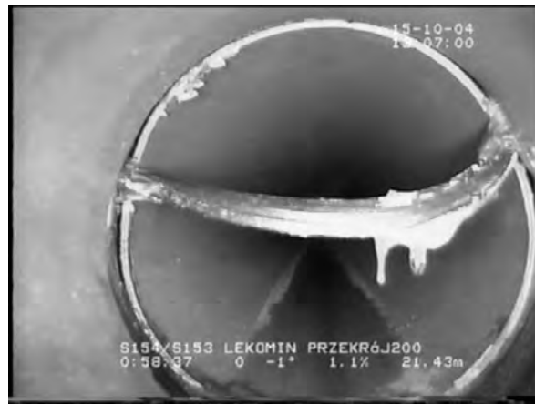
Fig. 17. The sealing that juts out from the place of pipe connection to the pipe interior
