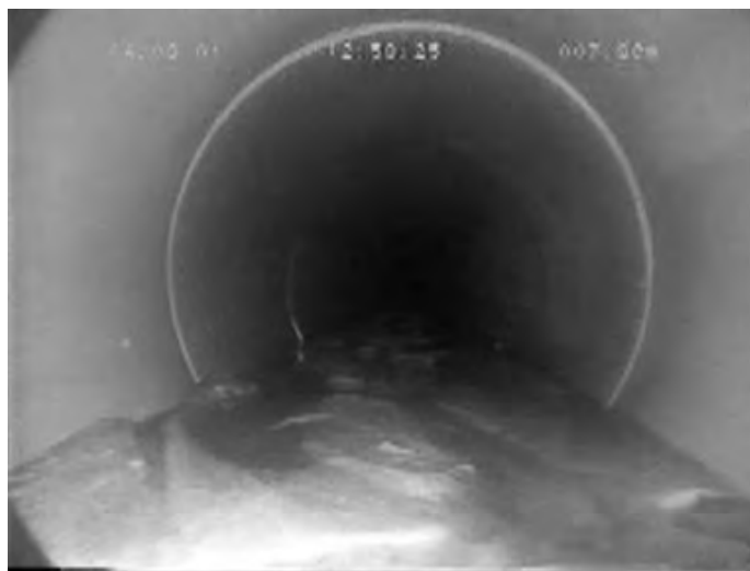
Fig. 10. The movable sediment, which was classified to 4th class of failures
